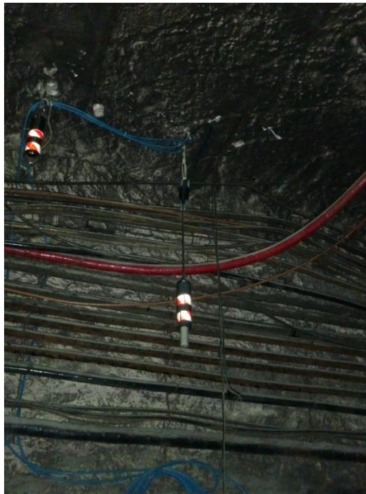
Figure 3: ultrasonic- and pressure sensors in the mine
