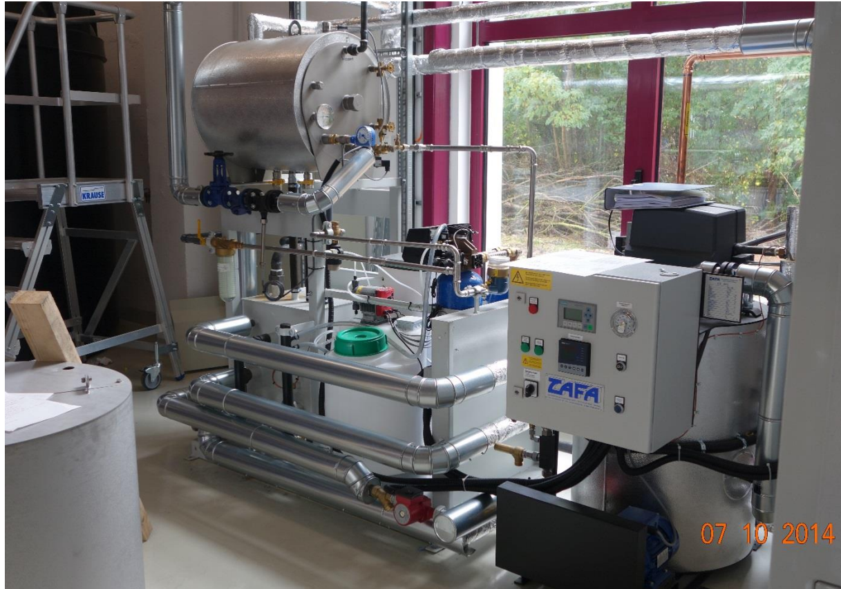
Steam generator (left) and evaporator (right)
