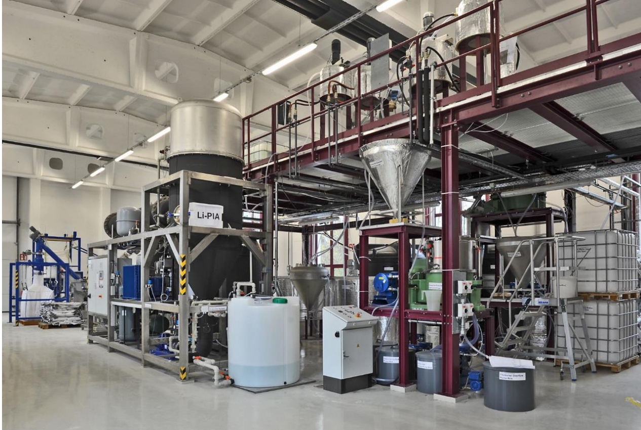
Total view lithium pilot plant (Li-Pia) with evaporator and crystalliser
