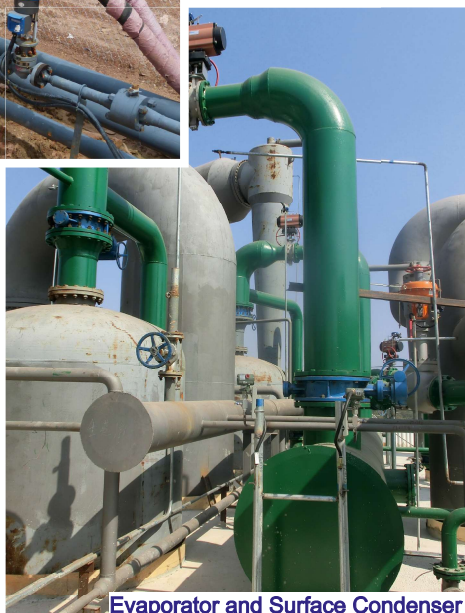
Evaporator and Surface Condenser
